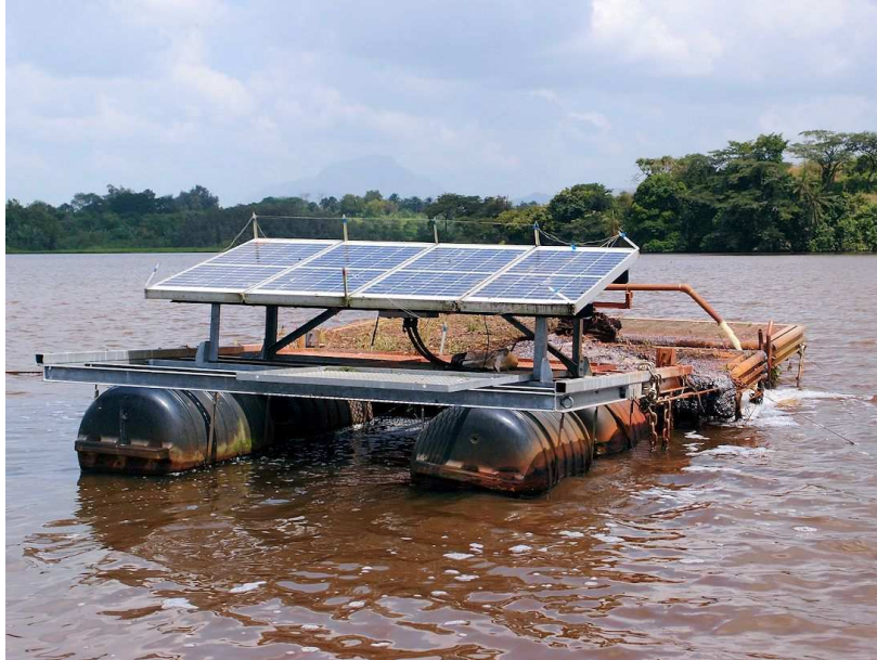
Photo 1: The solar power-driven deep water removal system (November 7 th , 2015)
